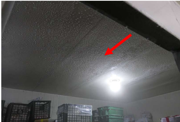
4/2 :冷凍庫天花板結露
